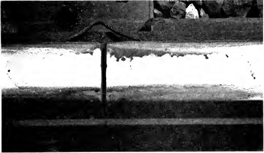
Fig. 2—Photograph of joint 11 showing porosity at weld junction of west rail.
